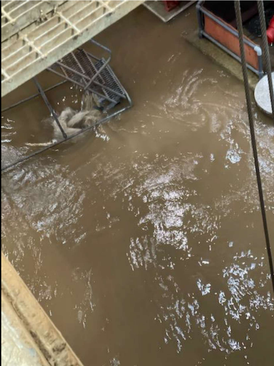
View from second floor looking down to flooding on the first floor.
