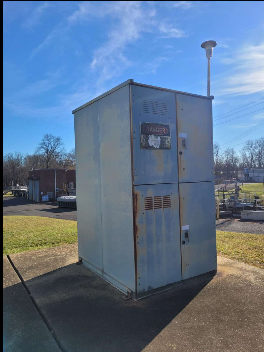
1 of 2 – 33,000 KVA Fuse Box
