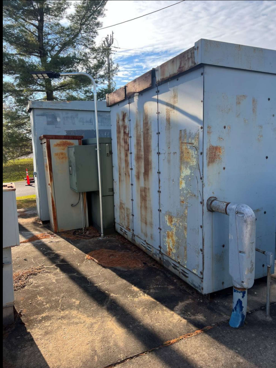
1972 Switchgear for 4160V
